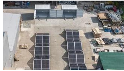
10mw photovoltaic cabinetized system for cement plants
