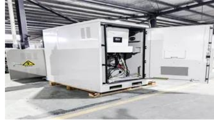
Container ESS 500kW/1053kWh
