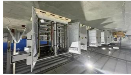
Niue Solar Photovoltaic Energy Storage System , ESAFETY SOLAR
