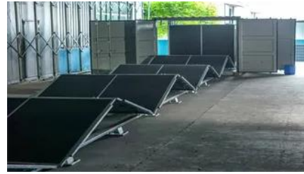
BESS: Battery Energy Storage System , Generac Industrial Energy
