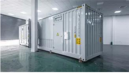
containerized battery storage , SUNTON POWER
