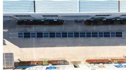
Warsaw Low Carbon Photovoltaic Energy Storage System
