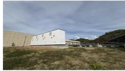
Energy storage high voltage cabinet structure
