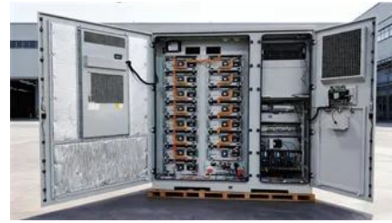
Kiribati communication base station wind and solar hybrid equipment
