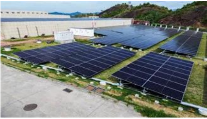
Galvanized square tube photovoltaic power generation bracket
