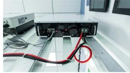
Mobile Solar Container Systems , Foldable PV Panels
