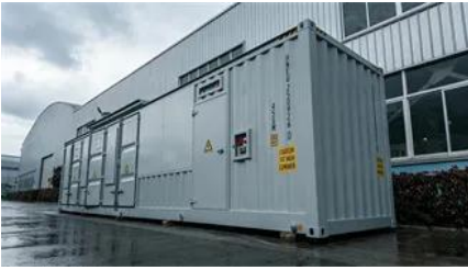
Battery Energy Storage in Port of Spain: Powering a Sustainable Future
