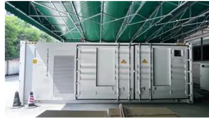
Rwanda 5G solar communication station battery energy storage
