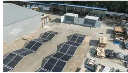
Solar container lithium battery station cabinet installation conditions
