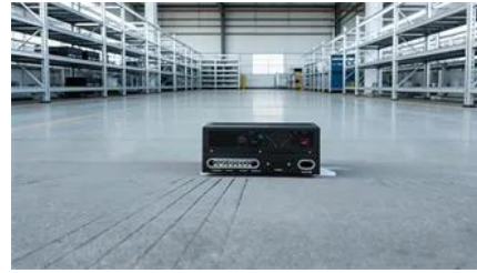
Site Battery Storage Cabinet, Base Station Energy Storage
