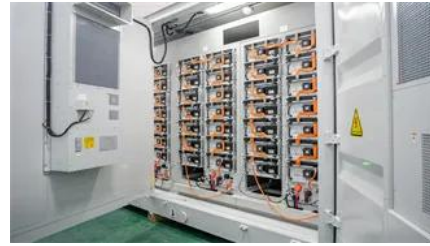
Somaliland solar container communication station inverter grid
