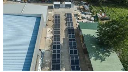
Communication base station solar and wind power generation
