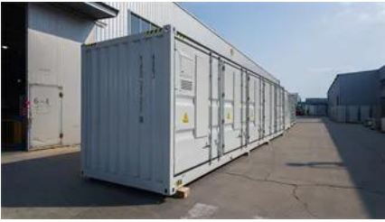
Outdoor Energy Storage System Cabinets , EPC Energy
