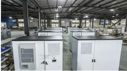
Uninterrupted power supply to solar container communication stations
